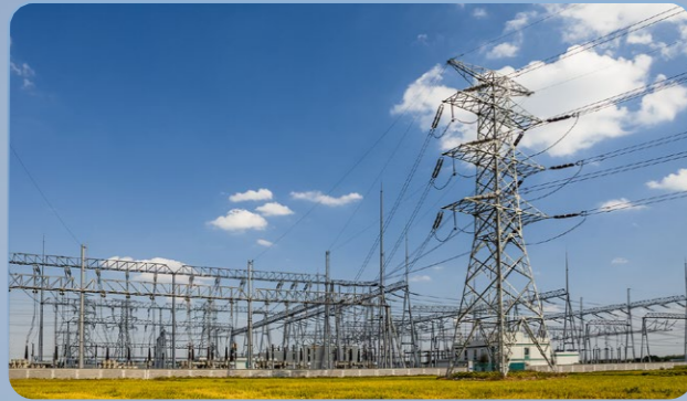
Intelligent peak-valley electricity utilization Save electricity costs
